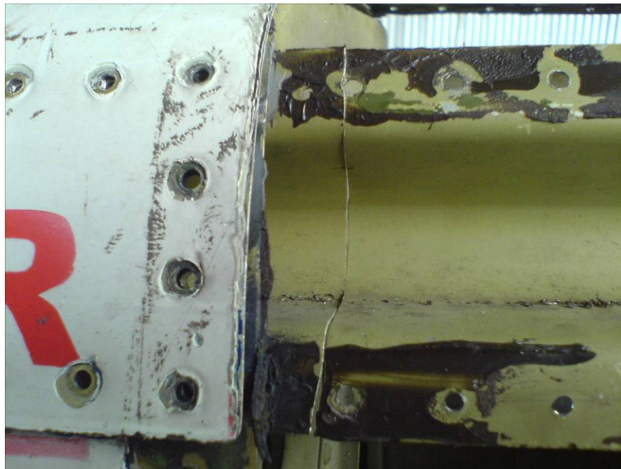
Figure 2 Cracked Longeron (upper skin removed) Aft of B.S.194.30
